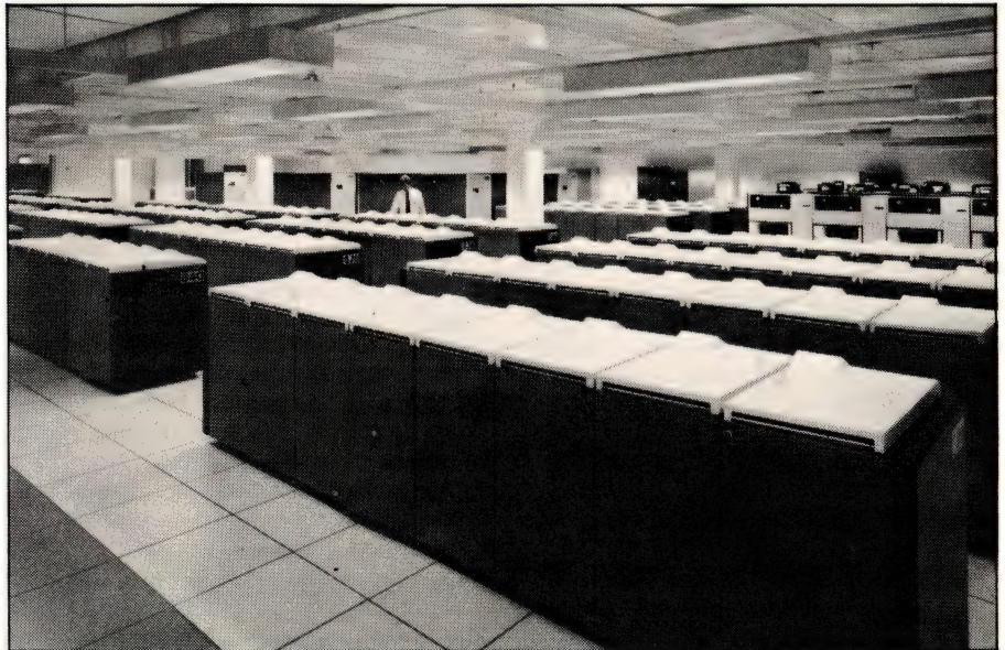
Computer power! The computing centre at IBM Australia's new Cumberland Forest (Sydney) headquarters has $80 million worth of hardware — including 80 gigabytes.
